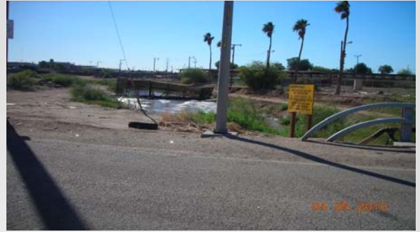
Above: Water level increased at the international boundary as a result of the lining damage in Mexicali.
